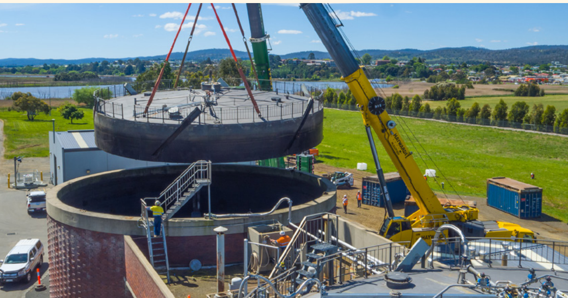
Ti Tree Bend Sewage Treatment Plant
