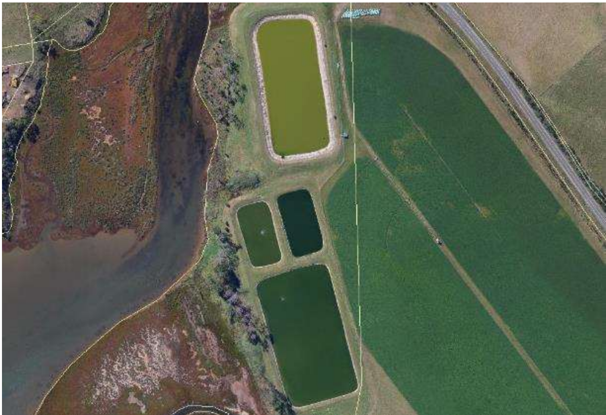
Figure 70-1: Triabunna Sewage Treatment Plant
